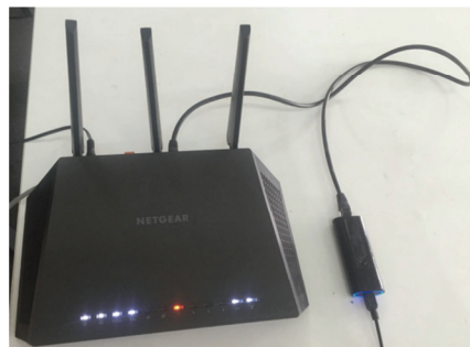
Fig. 5. The applied router and the smart gateway for connecting the air conditioners to the Internet.
